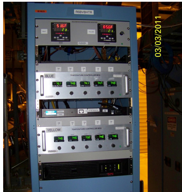
Figure 4: Installed Temperature Controller Rack System in a RHIC Service Building.
