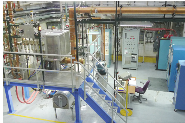
Figure 1: FPA at platform with ancillary equipment
