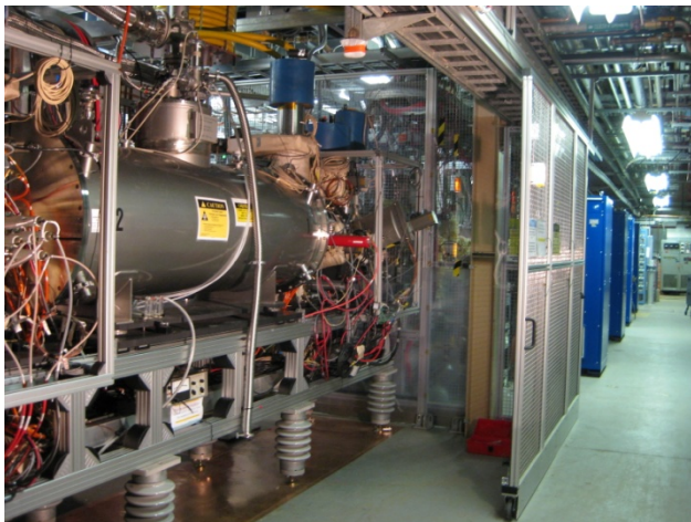
Figure 1: EBIS High Voltage Platform.
