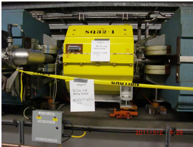
Figure 1: Tune jump magnet in the AGS tunnel.
