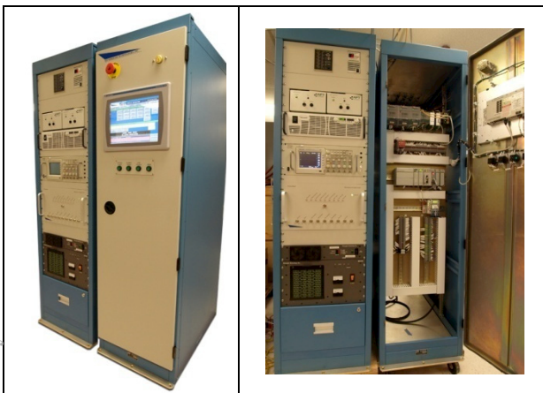
Figure 6: Controls racks for the 2 MW klystron transmitter.
