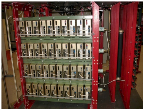
Figure 3: Switch plate array in the transmitter's modulator. The entire assembly is submerged in oil.
