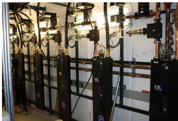
Figure 3: RF Distribution for six cavities. Large boxes are variable delay lines. Vector modulators are in front of lights.
