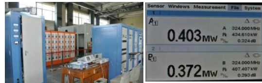
Figure 5: RFQ power source and its output power in test.
