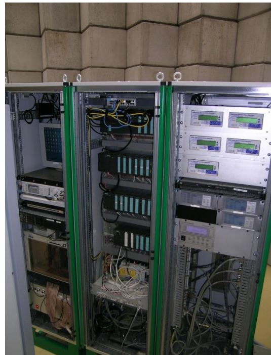
Figure 1: RFQ LCS Racks for Power Tests.
