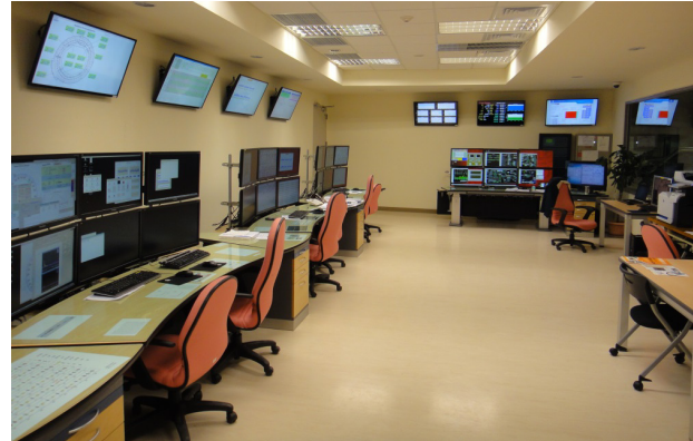
Figure 1: Console in the TPS control room includes multiple LCD screens and ready for use.
