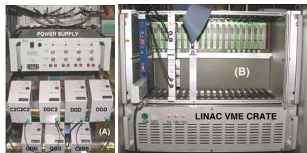
Figure 2: (A) A combination of 7 Group3 DIs services 8 RF Controllers and 16 stepping motors - C2: 8 ADC inputs -D: 8 analogue outputs - G: Logic drivers control up to 4 stepper motor; B: 24 digital channels, input and output. (B). Loops of DIs are controlled from a VME crate.
