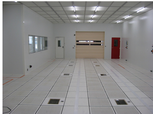
Figure 5: The new ISO4 cleanroom at CEA Saclay/IRFU.
