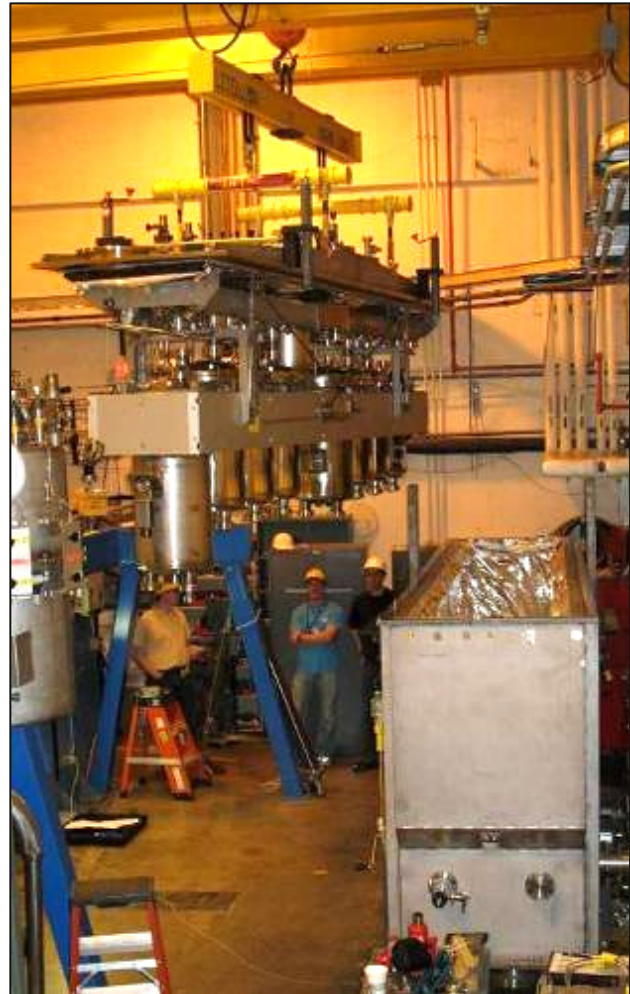
Figure 10: The lid/string subassembly is loaded into the cryomodule.
