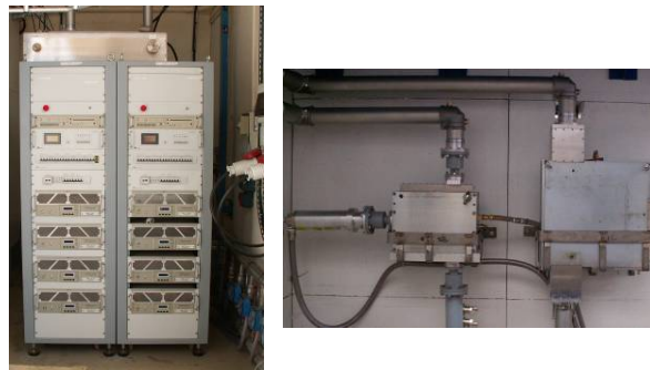
Figure 12: (left) two 10 KW combined to deliver 20 KW, (right) 10 and 20 KW circulators.
