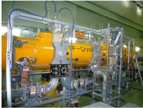
Figure 5: Installation of the cryomodule in the STF tunnel. Four input couplers were connected with the high power rf distribution system.
