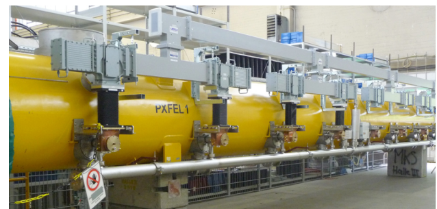
Figure 13: Module PXFEL1 with XFEL-type non-equal pre-adjustable binary RF power distribution.
