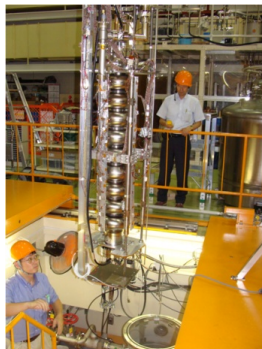
Figure 4 : Installing 9-cell cavity to cryostat
