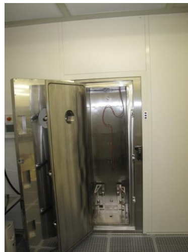
Figure 4: View from inside ISO 4 area on the loading area of the 120°C in-situ heating chamber.
