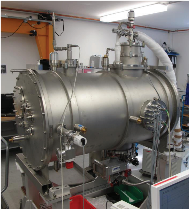
Figure 2: Photograph of the new SRF gun cryomodule.
