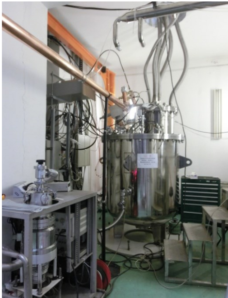
Figure 9: The cryomodule of Spoke012 with cavity in it.
