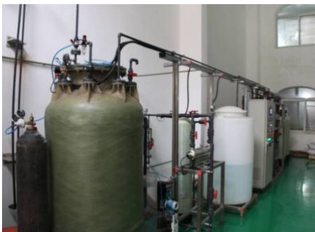
Figure 4 : UPW supply system at Daxing base.
