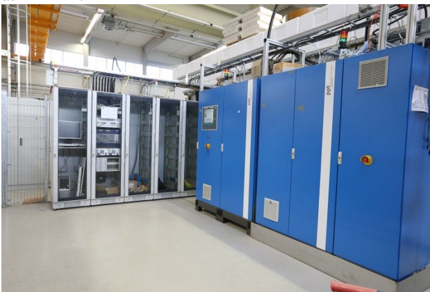
Figure 3: LLRF racks (left) and the 3.9 GHz klystron and modulator racks in the XATB1 module test cave.
