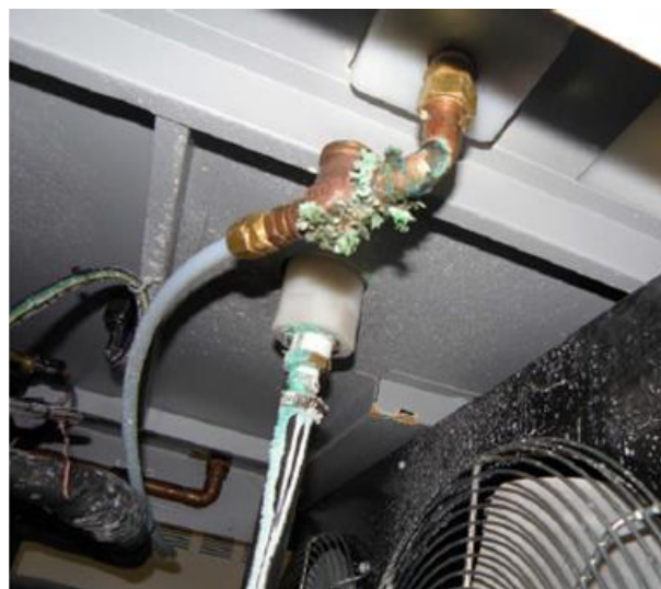
Figure 4: Corroded chiller fittings on AES Baseline tool.
