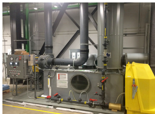
Figure 2: Toxic gas scrubber unit.
