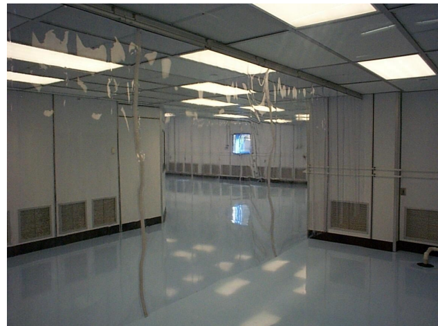
Figure 1: The new class 100 cleanroom.
