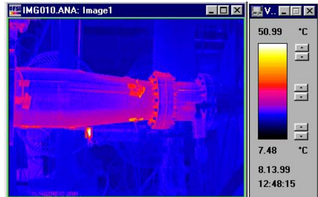
Figure 18: Thermal image of the tapered section, 300 kW
