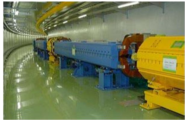
Figure 11: Installed MR magnet.
