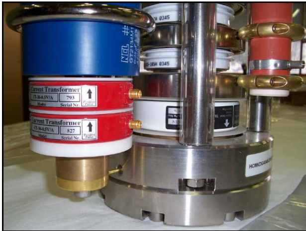
Figure 2: Re-trigger CTs in the main discharge switch.
