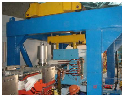
Figure 5: The dipole installation.
