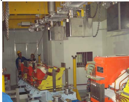
Figure 4: The vacuum chamber installation.
