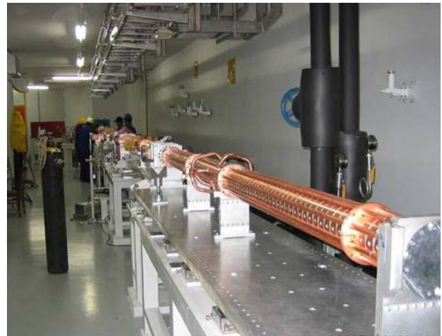
Figure 3: The SSRF linac under installation, January 2007.
