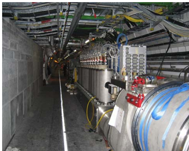
Figure 15: Current feed boxes.
