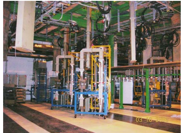
Figure 12: Two 300 kW klystrons with circulators and loads.
