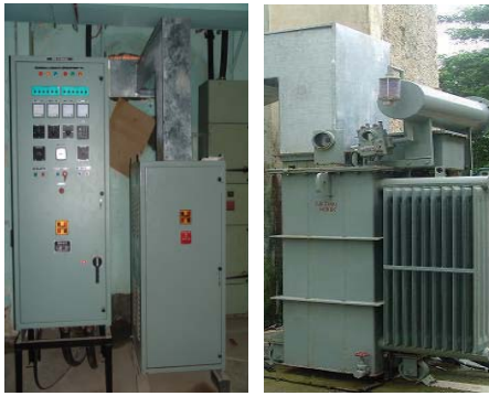
Figure 2: Anode power supply and its transformer unit.
