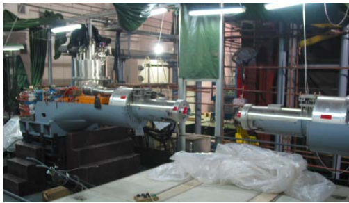
Figure 9: SCQ's and some warm magnets installed in IR.
