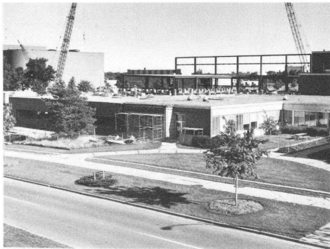
Fig. 20: A view of the office addition of approximately 16,600 square feet is shown. The addition will include a seminar room, eleven new offices, plus a large open office area. An additional 3500 square feet of the existing building has been modified.
