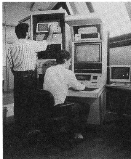
Fig. 1 - The operator console in the main control room
