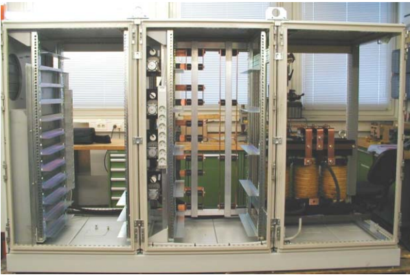
Fig. 3 Internals of the electronic racks
