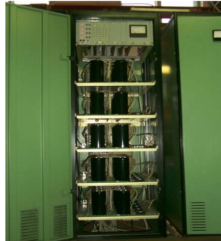
Figure 4: Housing 19-inch rack for the electrolytic capacitor ("B43458" type) storage bank.
