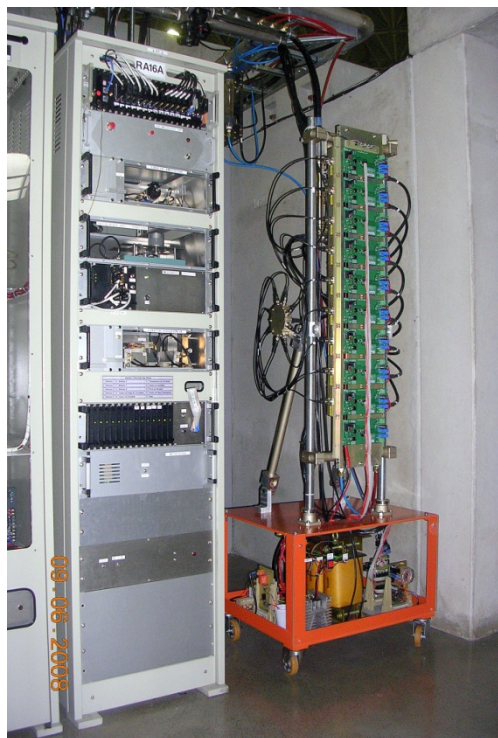
Figure 2: 2.2 kW amplifier Installed in the Booster Injector
