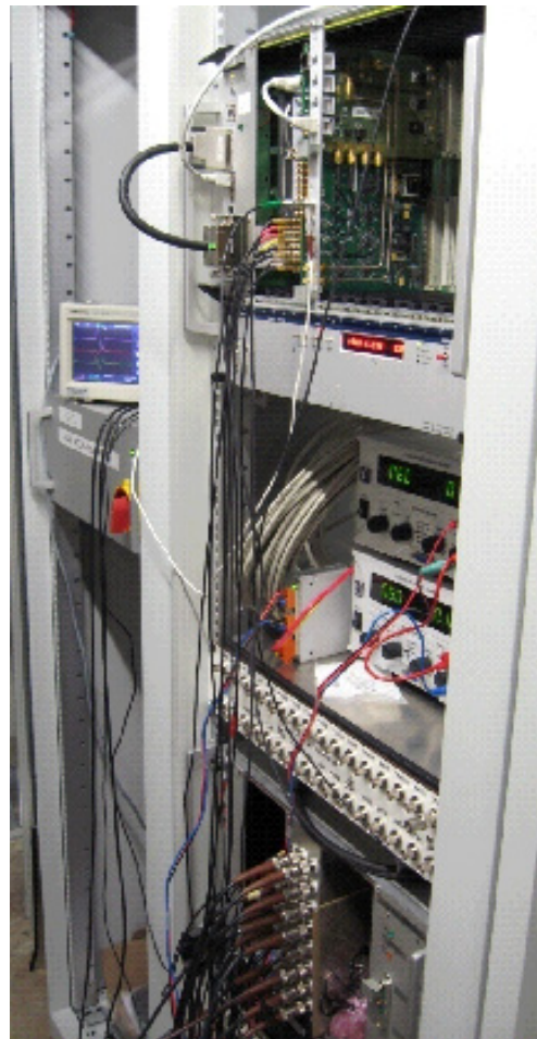
Figure 4: Piezo control system installed in FLASH.
