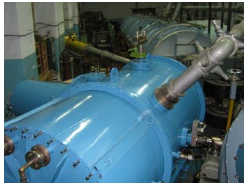
Figure 10: New pre-stripping section PSS-4 in the MILAC main hall.
