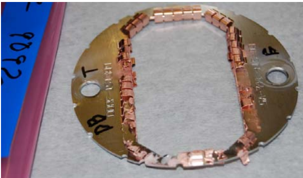
Figure 8: Melted omega seal of the 9092-flange.
