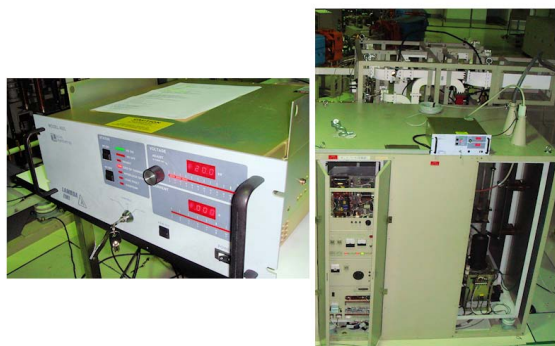
Figure 2: High frequency switching PS for the linac klystron under testing (left) and after installation atop the old HV PS (right).
