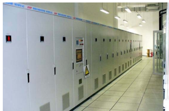
Figure 7: The dynamic power supplies for SSRF booster
