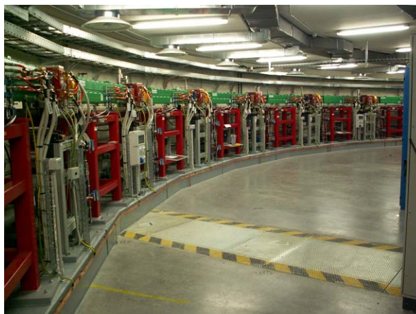
Figure 2: Booster Arc West.
