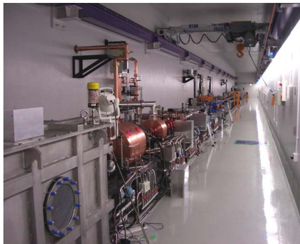
Fig. 2: Tunnel view in SCSS test accelerator.
