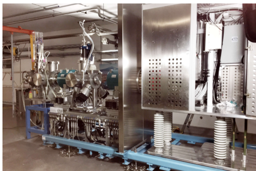
Figure 5: IS and LEBT installed in the ESS linac tunnel.
