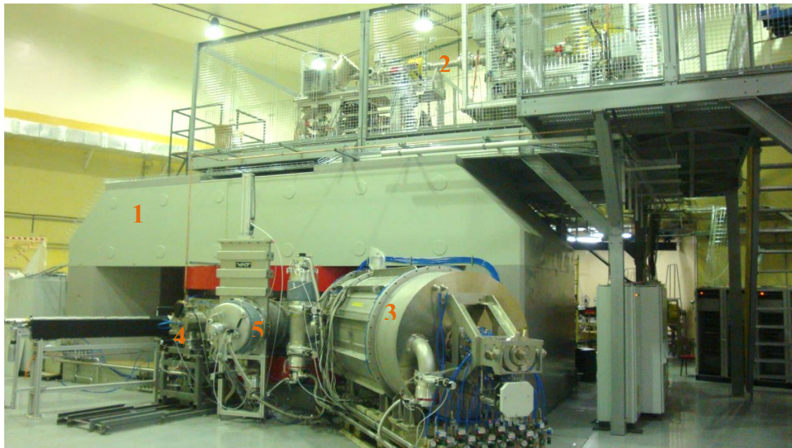
Figure 4: The new DC-280 cyclotron, where: 1- Main magnet, 2- HV injection system, 3- RF resonator, 4- Flat-top resonator, 5- Vacuum pumps.
