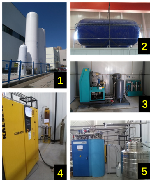
Figure 3: Cryogenic test station High pressure helium storage tank (1), Air bag (2), Compressor (3), TCF10 (4), Liquid helium dewar (5).
