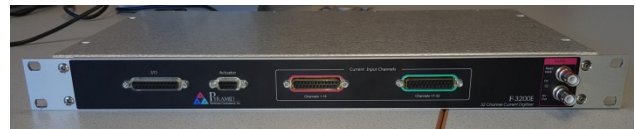
Figure 13: The grid electronics Pyramid F3200E that will be used has arrived at NTG and is currently prepared, tested and commissioned.
