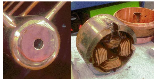
Figure 2: Drift tube of Alvarez section, as installed (left); opened drift tube with defective quadrupole lens (right).
