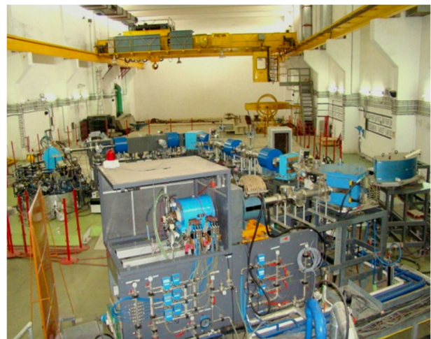
Figure 2: 14GHz ECR ion source and injection beam line.
