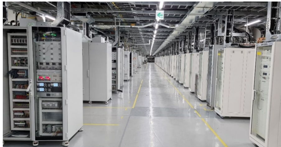
CM/Cryogenic Control Rack and SSPA
